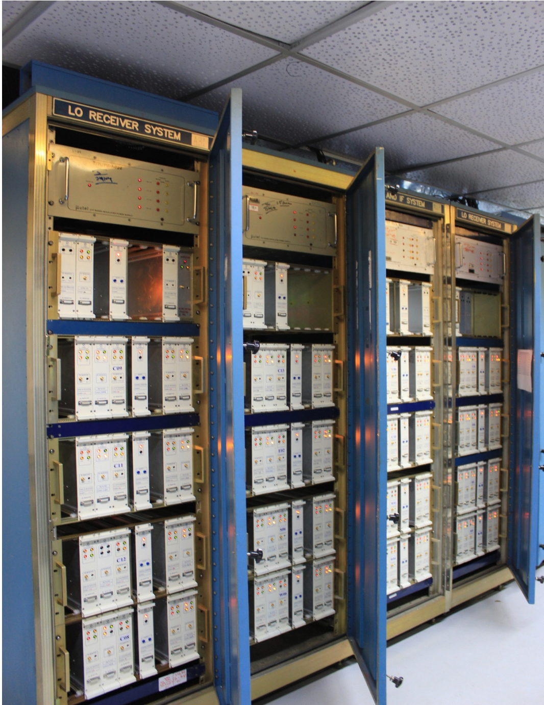
GAB System Rack – Front Side
