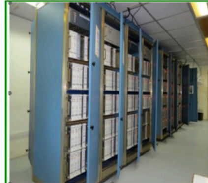
Fig 1: GAB System at Receiver Room.
