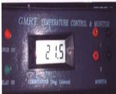
a) Temperature Monitoring Unit
