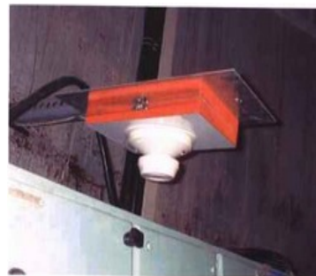
b) Smoke & Fire Alarm Sensor
