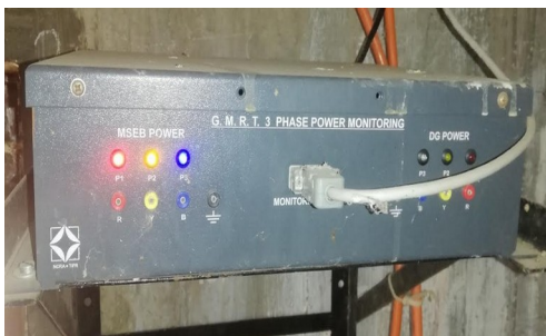
c) MSEB/DGSET power monitoring Unit
