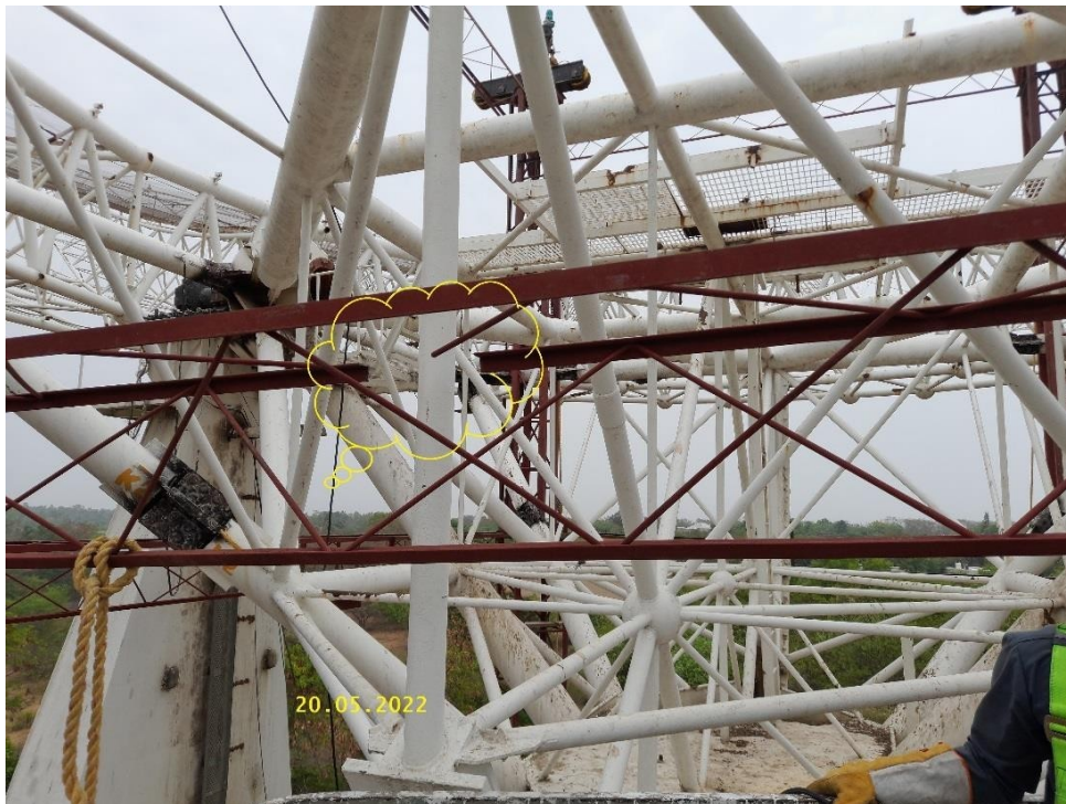
Girder fouling on Pin sector
