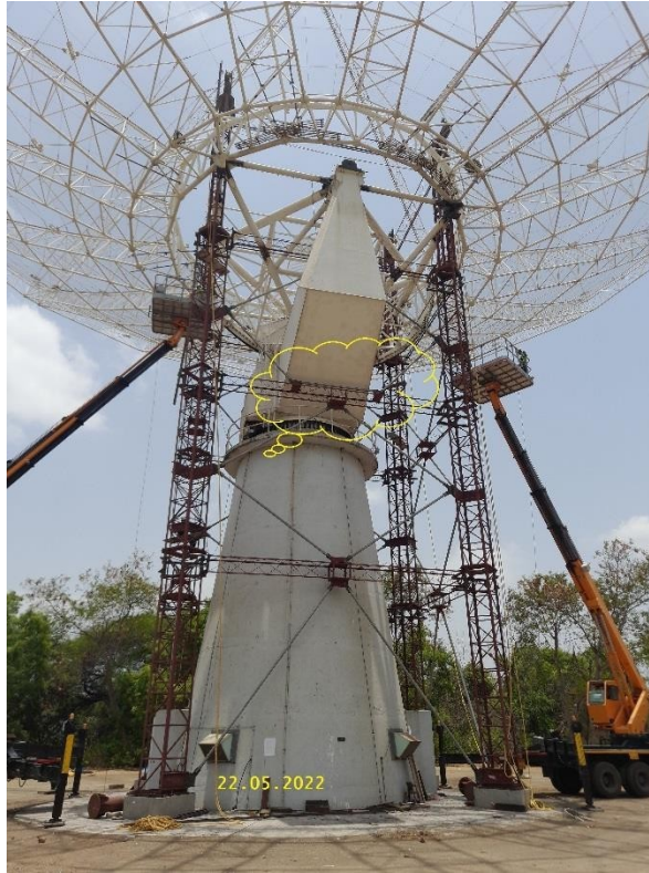
Bracing members are fouling @ Yoke body
