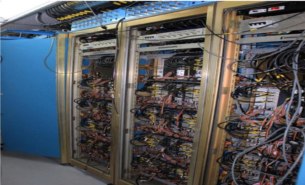
GAB System Rack – Rear Side
