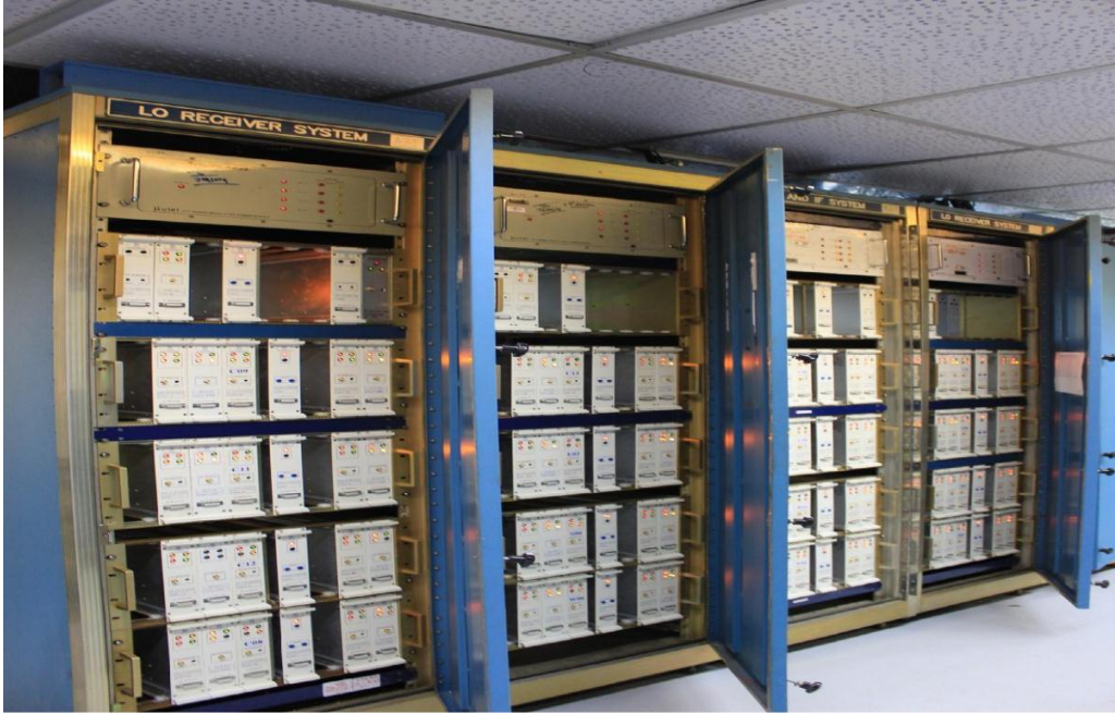
GAB System Rack – Front Side
